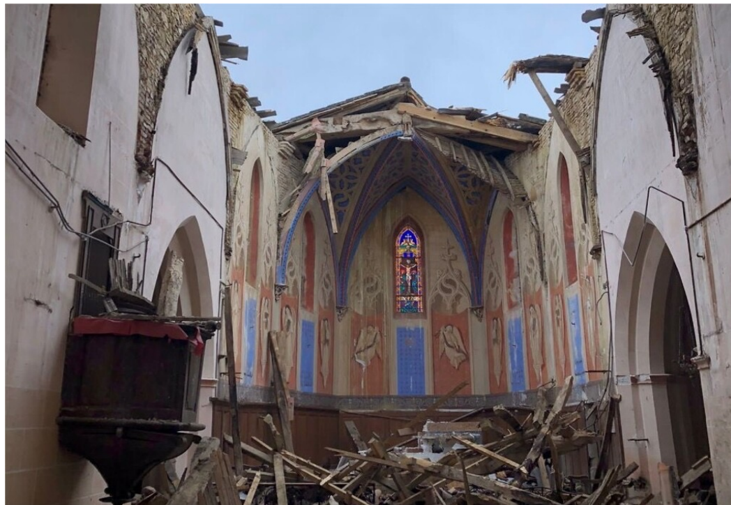
Roof of Monferran-Savès Church in Gers (France) collapsed in Jan. 2024.
